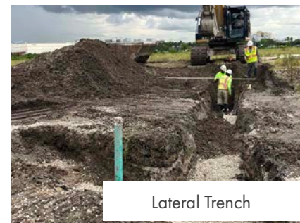
Lateral on Sanitary Sewer Main Line
